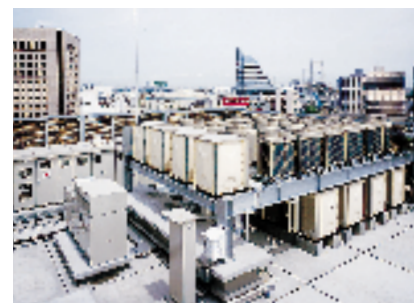
Heat pumps operated by ice thermal-storage systems (Shibaura building)
