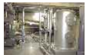
Recycling facility for general service water (Koishikawa building)
