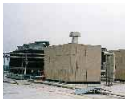
Absorption refrigerating machine
