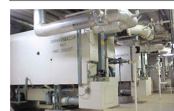
Absorption refrigeration machines
