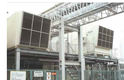
Cogeneration system at Toppan Graphics Co., Ltd.
