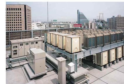
Heat pumps operated by the ice-thermal-storage systems (Shibaura building)
