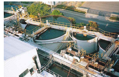
Wastewater treatment facility/coagulative precipitation tank
