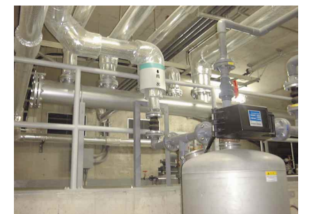
Rainwater pipings (Toppan Koishikawa Building)
