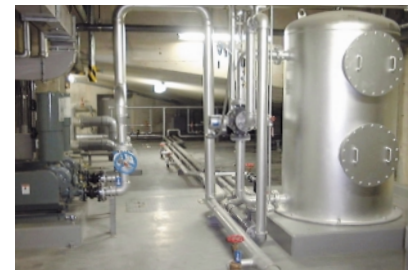
Used-water recycling facility (Toppan Koishikawa Building)
