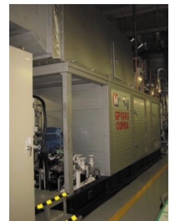
Cogeneration system at Fukuoka plant No.1
