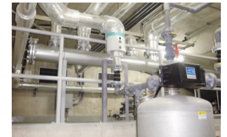
Rainwater piping (Toppan Koishikawa Building)
