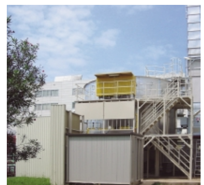
Waste gases combustion facility
