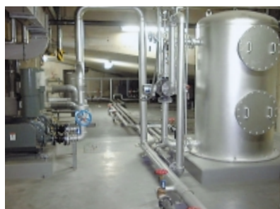
Used-water recycling facility (Toppan Koishikawa Building)
