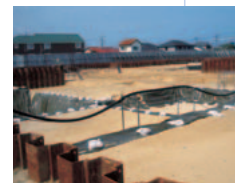
The site of soil restoration work. Contaminated soil is removed and replaced with new soil in each block.
