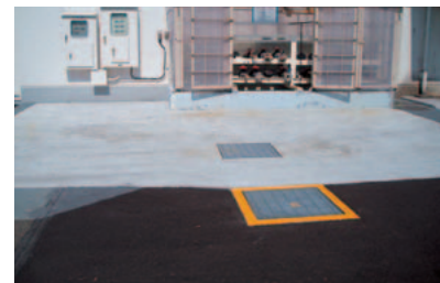
In case of chemical spillages in the truck loading entrance, a pit has been dug to prevent the leakage spreading around or even escaping the area. (Toppan Electronics Fuji Co., Ltd.)
