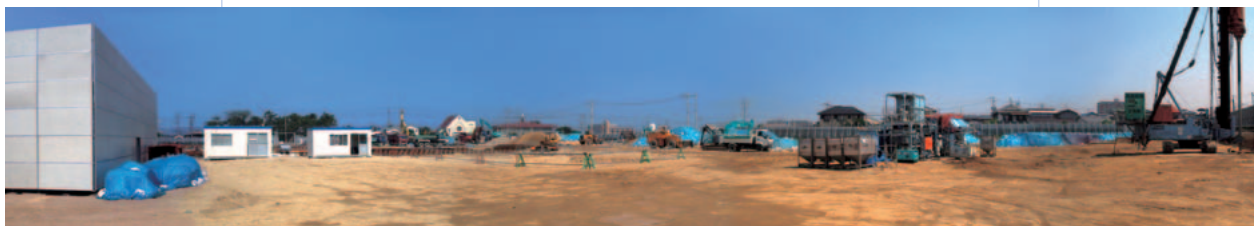
A complete view of the soil restoration and groundwater purification work site (left: the groundwater purification facilities; right: VOCs decontamination work)
