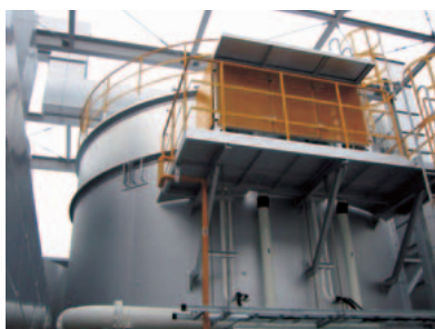
Gas emissions processing equipment (Fukuzaki plant)
