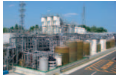
Wastewater recycling system (Mie Plant II)
