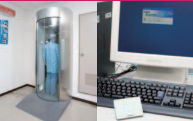
Left: Entrance gate secured by a personal authentication system and double door to restrict entry to authenticated persons only
