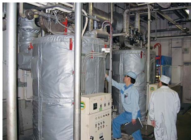
Boiler insulation jacket to minimize thermal loss
