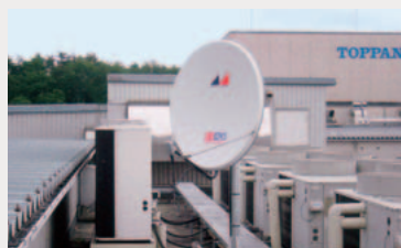
Parabolic antenna to receive Earthquake Early Warnings by radio
