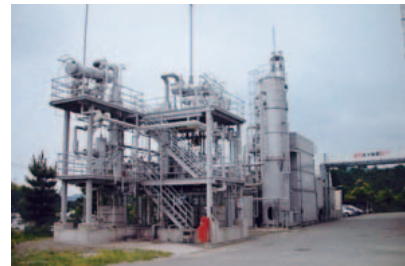
Equipment for recovering solvents (Fukusaki Plant)
