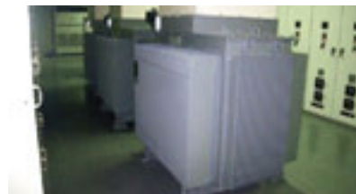
Highly efficient power transformers (Sakai Plant, Toppan Electronics Products Co., Ltd.)
