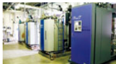
Fuel switchover for boilers (Ranzan Plant, Toppan Communication Products Co., Ltd.)
