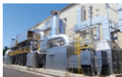
Effluent gas-treatment equipment (Fukaya Plant)
