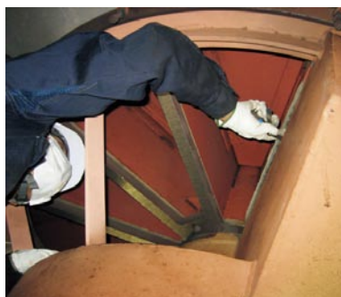
Inspection of effluent-gas treatment equipment
