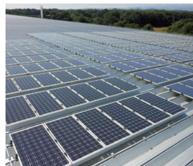
Solar panels (Fukaya Plant)
