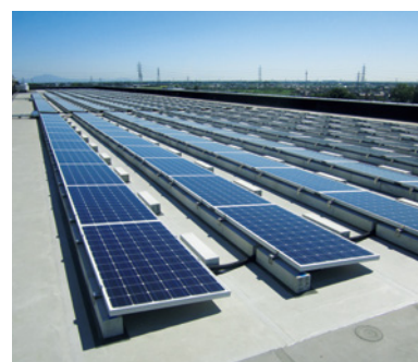
Solar panels (Experiment Center, Toppan Technical Research Institute)
