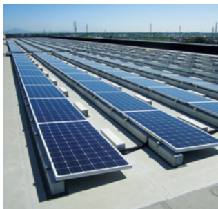
Solar panels capable of generating approx.150 kW of electricity installed on the roofs of Fukaya Plant and Toppan Technical Research Institute
