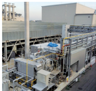
Cogeneration system introduced in Gunma Central Plant following its launch into full-fledged operation in May 2015
