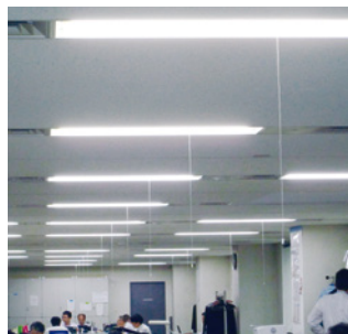
Switching from mercury-vapor lamps and fluorescent lights to LED lights. All of the fluorescent lights used at the head office have been replaced by LED lights.
