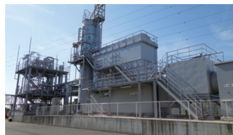
Facility for recovering solvents (Gunma Central Plant)
