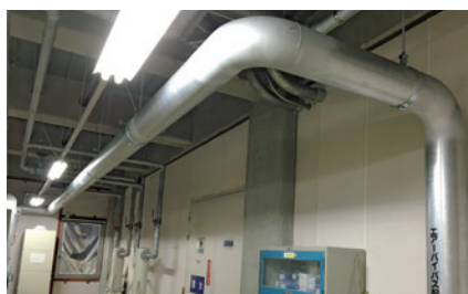
Air piping rearrangement (Ranzan Plant)
